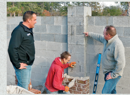
Clint Bell (left) and Russell Huntley (right) on the site of the Living Dunes community under construction in Myrtle Beach. East Coast Masonry & Stone is handling the brick and block for this CRG Companies' project.
