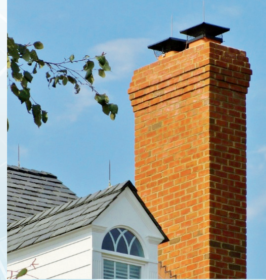
Notice the two air terminals (ATs) on the roof line & another two on the top of the chimney. These are the only visible components that can be seen from the ground.
