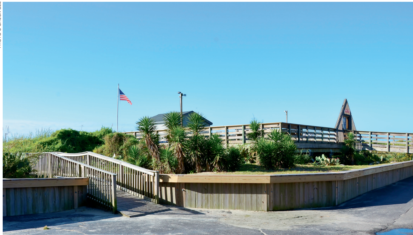
In addition to the pier boards and bench replacements, CCCG also constructed a new pier gate and sea wall-cap.
