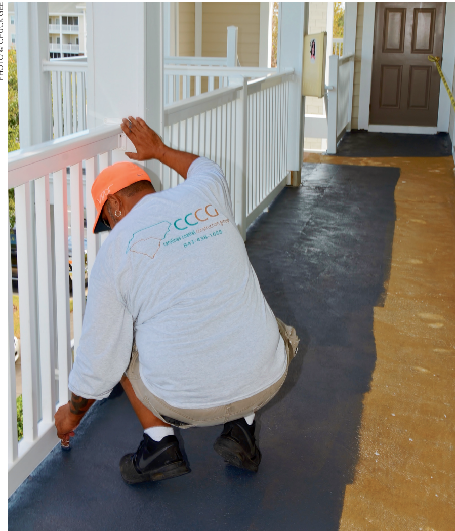
J.P. Pollio (crew leader) applies a water tight membrane to an exterior carpet replacement project in the Carolina Forest area. The membrane installation is applied much like a roof coating in multiple coats and thickens as it dries to provide a rubber like membrane.
