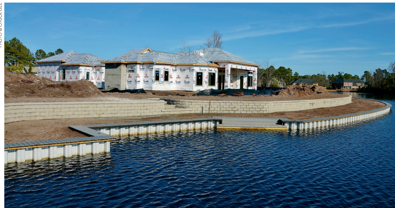
CHC has completed the largest seawall in Plantation Lakes. “We also build kayak docks so homeowners can paddle from the lake straight onto the dock in their backyard”, says Jeff Chestnut.
