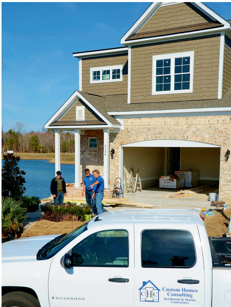
Layne Harris (right) & Steven Quickery (middle) explain the layout of the landscaping package to be completed to new homeowner, Chris Tobin, in front of the home of Chris & Cindy Tobin under construction at Waterway Palms in Myrtle Beach.
