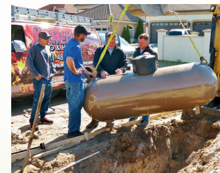
Palmetto Patio & Hearth / Palmetto Propane owners, John Gaddy (2nd from right) & Stevie Bryant (far right) discuss the plans to bury a propane tank for a recent project.
