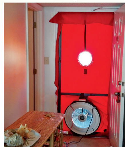
Carolina Cool performs the blower door test which allows the technician to find any areas of leakage.
