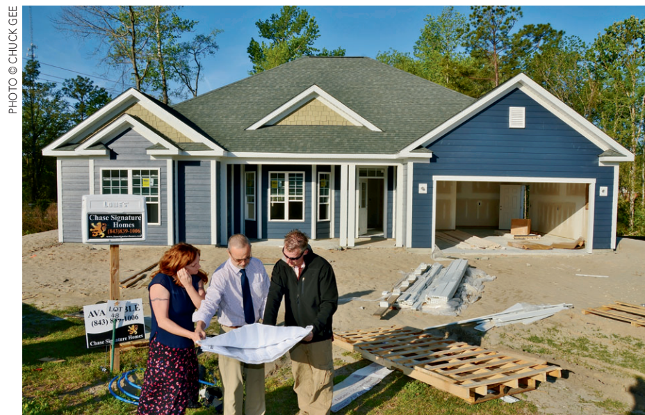
Syd Chase (middle), Julie Chase (far left) &amp; Aaron Bartlett (far right) review a set of plans for one of their homes under construction in Rivers Edge Plantation.
