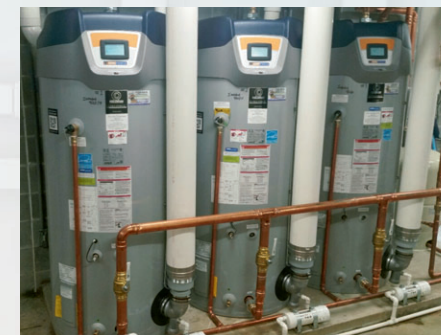
Carolina Cool has the capability to handle the smaller residential jobs, as well as the larger commercial jobs.
