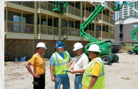
Contract Exteriors was responsible for replacing all of the decking on this ocean front condo complex in North Myrtle Beach.
