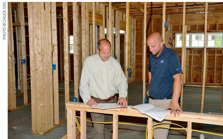
Stephen Dean (left), area manager for the Myrtle Beach division, and Richard Beck (right), project manager for the Myrtle Beach division, review the plans in a home under construction in the Indigo Bay community.
