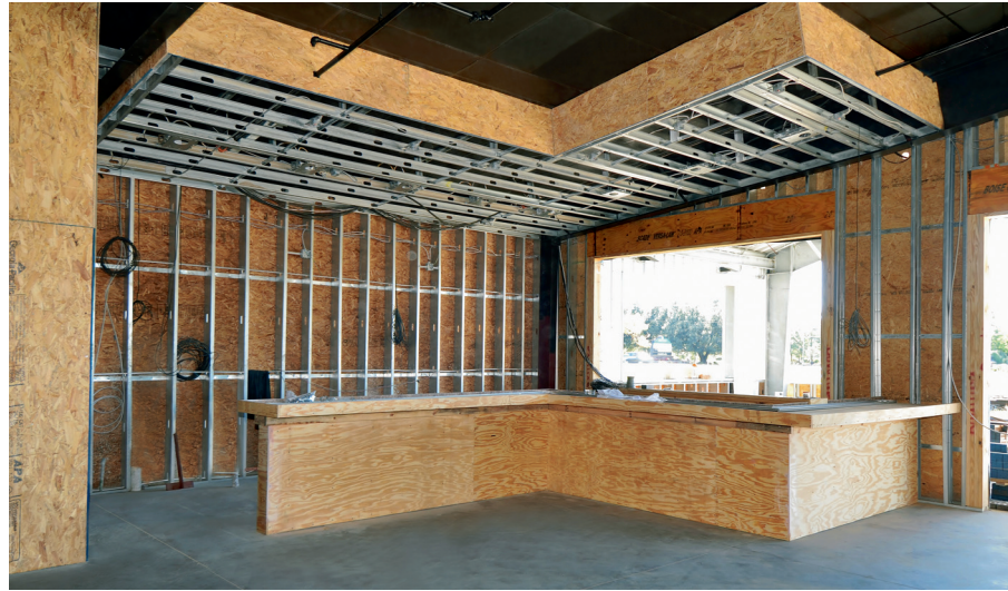
A bar area @ 810 in Conway while it was under construction. This bar will serve the exterior seating and features a soffit that follows the bar layout which was eventually covered with reclaimed wood. This bar that opens to the exterior seating was finished with a concrete top, OSB and copper laminate facing.
