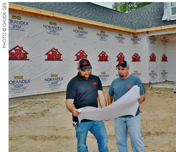
Roy Coffin (left) reviewing plans with custom home project manager, Joshua Coffin, on the site of a custom home under construction on one of BRB's one acre lots in Conway.
