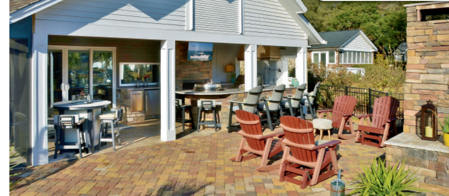
Jon Harrah was responsible for completing the total remodel/renovation of the rear of Lisa Phillip’s home in Mt. Gilead. An exterior wall needed to be added on one side (with matching stucco) so the roof could be extended over the space (with matching shingles). The design included a hibachi grill, sink, two refrigerators, lighting, and an overhead fan. Travertine was used on the floor. “Jon is a great contractor and I would highly recommend him. He did a beautiful job and fulfilled everything that was requested in a timely manner”, said Lisa.
