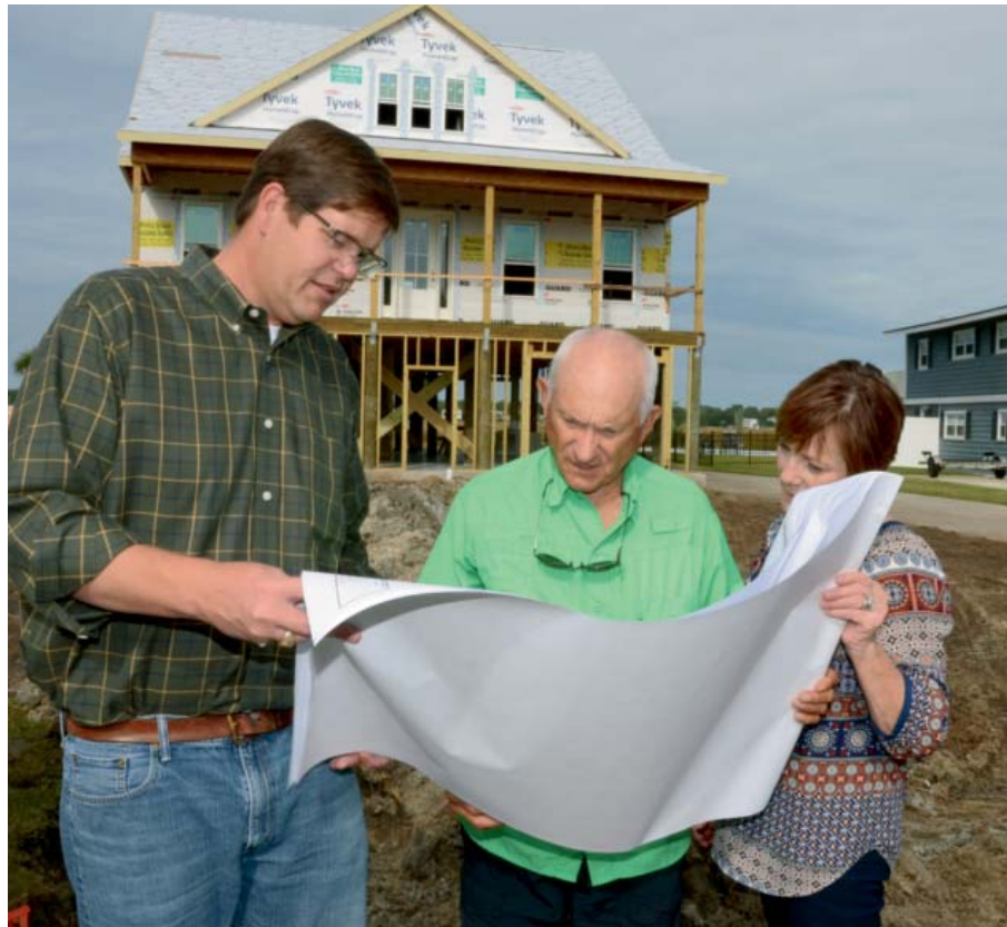
Drew Hanna (left) reviews the plans with homeowner's Woody & Nancy McKay in front of their home under construction in Garden City, SC. "We're pretty much building the same five bedroom house we had at Collins Creek Landing. We loved the layout and asked Drew if he could do it on 15' pilings." While still living at Collins Creek Landing Woody and Nancy watched 8 or 10 houses being built by Port City Homes and were impressed with their process. Woody said, "It was one crew after another. There was never any downtime. I thought, 'that's the kind of guy I want to build my house.'" Woody said, "We're just crazy about Drew and his family."
