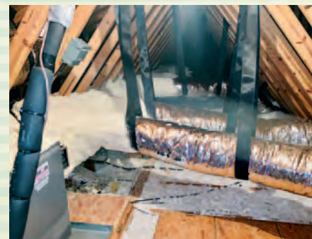
DeLuca emphasizes the highest quality company standards with his installers / service technicians. "I want them to look at every job as if it's going to be on display for everyone to see, which it is," says DeLuca.
