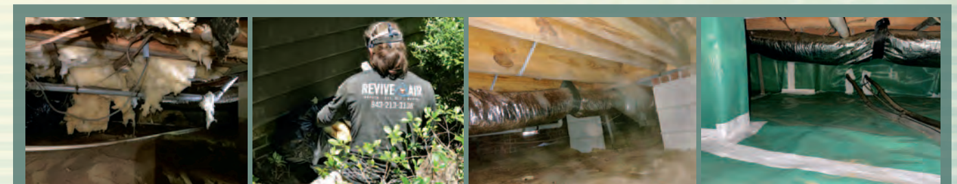
Revive Air was hired to remove all of the existing insulation & seal the crawl space under this residential home in Myrtle Beach.
