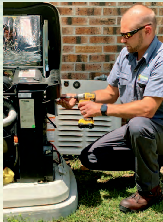
A Carolina Cool service technician performs maintenance on a residential standby generator.
