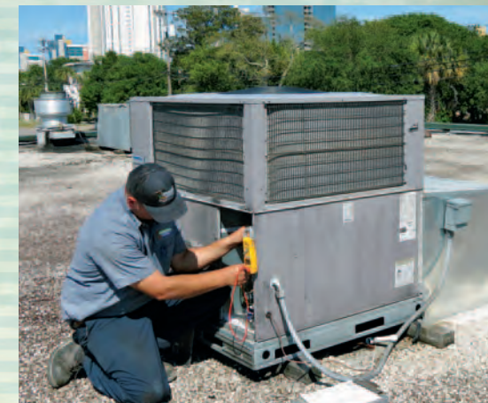
A Carolina Cool service technician performs maintenance on a rooftop unit @ a Myrtle Beach restaurant.
