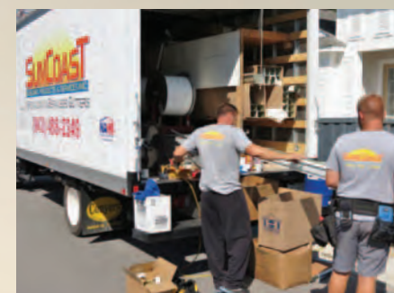
Darryl Hill (left) & Zeb Hill (right) measure and cut the custom gutters for a project in Ocean Isle Beach, NC.
