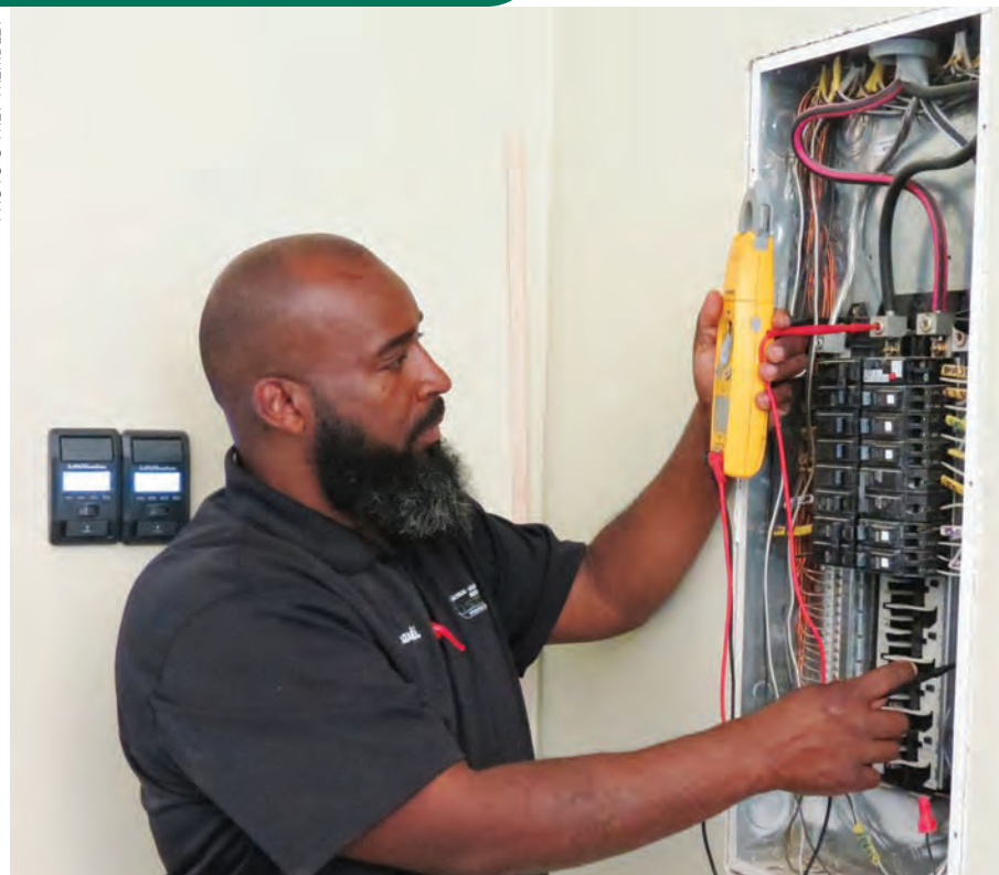
Electrical was one of the first services offered by Trusted Home Services back in 2017.
