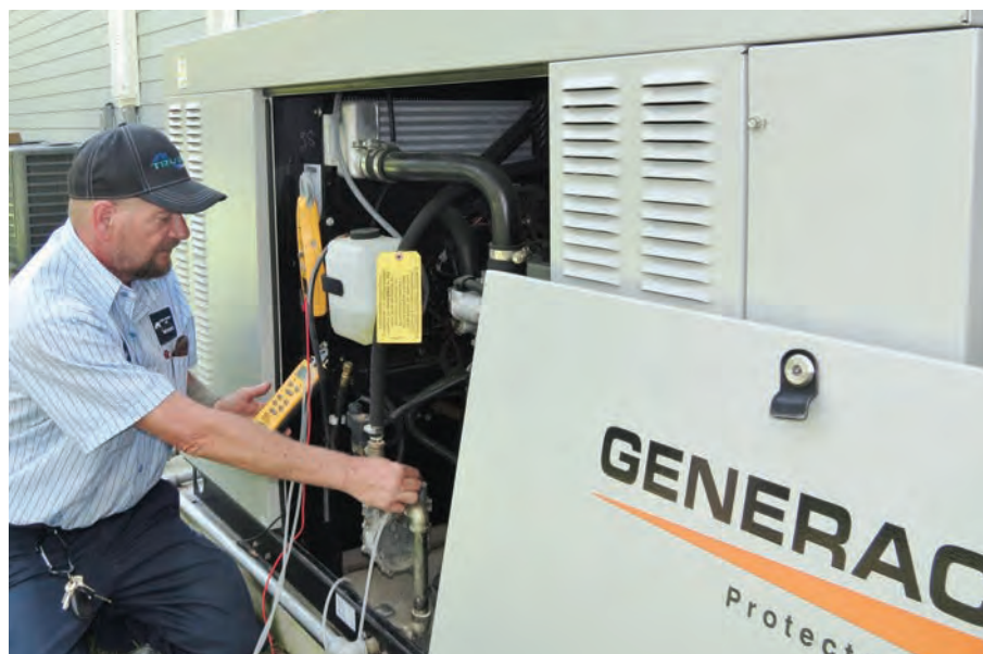
Generators are extremely popular in this coastal market & Trusted Home Services installs & provides maintenance for them throughout the area.
