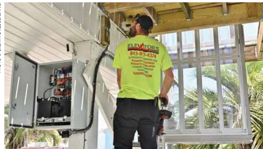
Licensed and certified Elevators Plus technicians are always available to ensure units are in proper working order.
