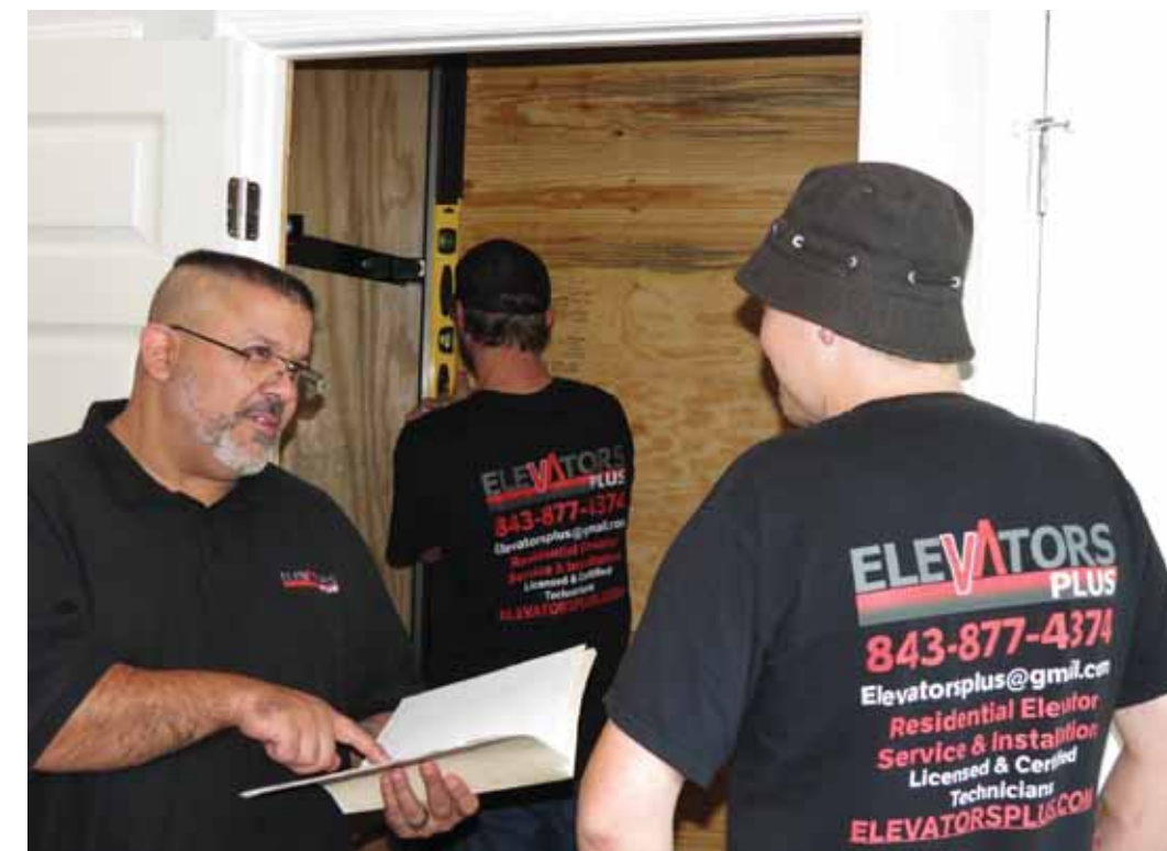
Elevators Plus project manager, Alex Morales, ensures a seamless installation from start to finish.
