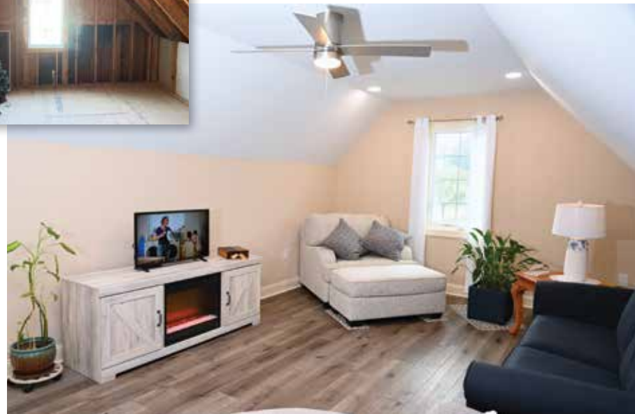
Jim Doring first met Clemons a decade ago, when Clemons was the project manager for their new home, stayed close over the years, and reached back out to him recently to help renovate his bonus room. "When we had the house built, we didn't have the money to finish the bonus room, so he came in and made it into a beautiful room," says Doring. "He's a great person, very personable, and he's just very in tune with things."
