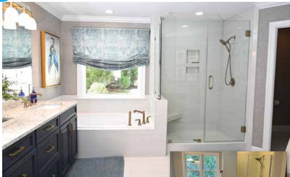
The master bathroom in the residence of Cyndi Moran is yet another example of Clemons and his team’s many talents. Carolina Bays replaced her roof and renovated her primary bathroom, installing new flooring, light fixtures, new cabinetry, replacing a window, and expanding the shower. “They did a great job with coordinating all of the subcontractors and everything,” says Moran. “It just made it really easy for me. I definitely would hire him again because there were no problems at all, and with any questions I had, he was always available to help.”
